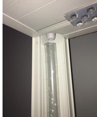
Drain tube disconnected
