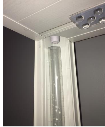
Drain tube disconnected
